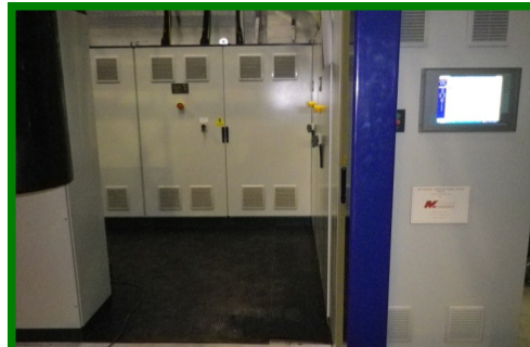
New PET air compressor control panel
