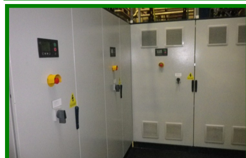
3 off 300kw Inverters for PET air compressors
