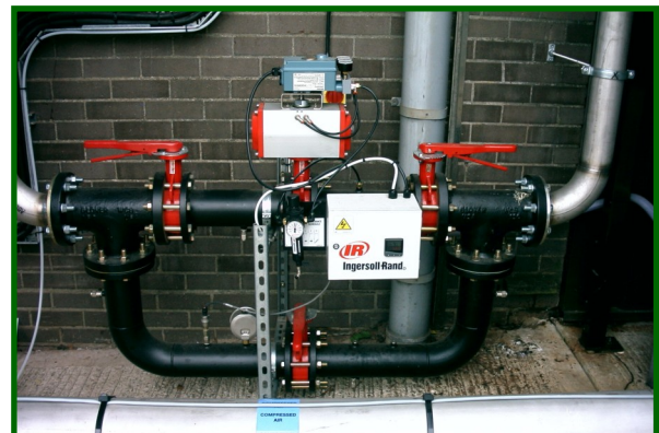
Intelliflow valve installation
