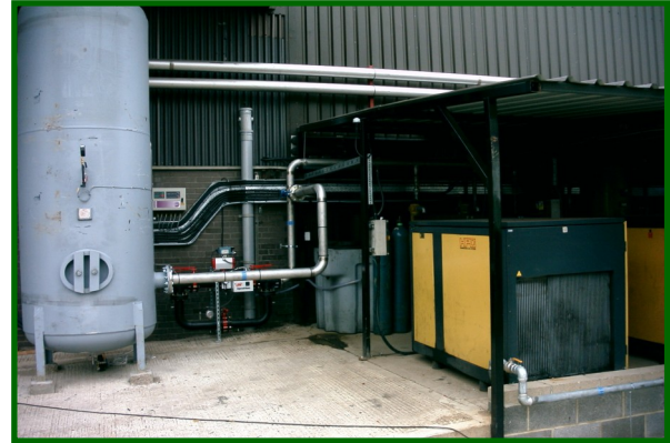
5000 litre dry storage tank
