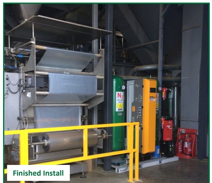
Nitrogen Generation Skid System
