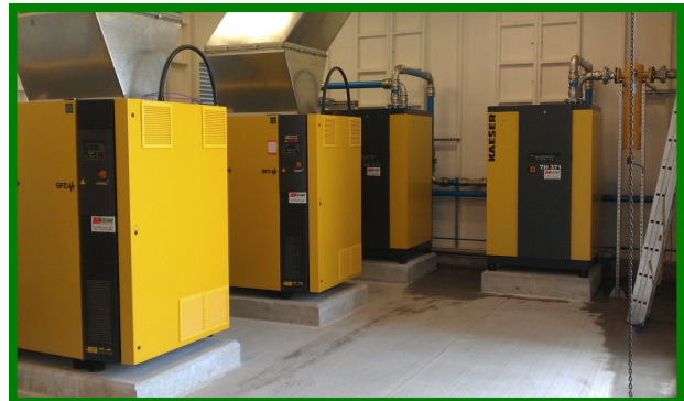
New HPC compressor plantroom installation
